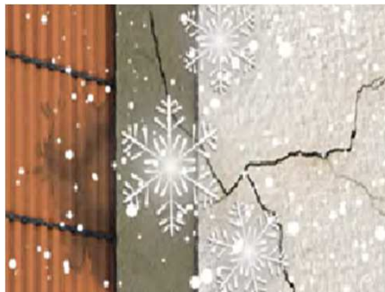
Protect against frost
